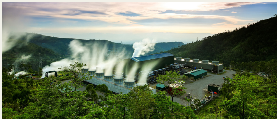
Energy Development Corporation's Geothermal Plant in Leyte, Philippines
