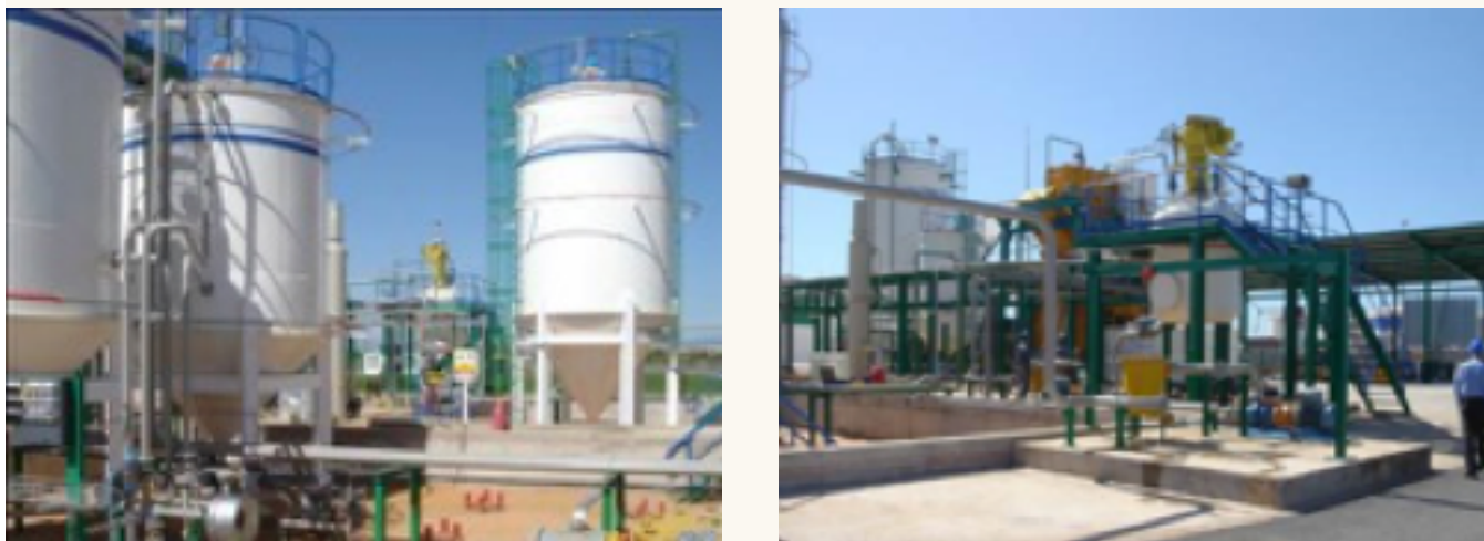
Figure 38: Example of Facilities for Liquid Alternative Fuel Preparation
