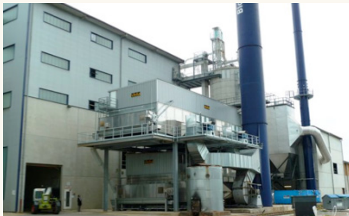
Figure 25: Belt Dryer Using the Excess Exhaust Gases from Kilns
