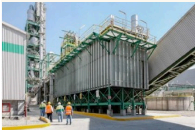
Figure 4: Storage and Injection Facility for Solid Wastes in Mexico
